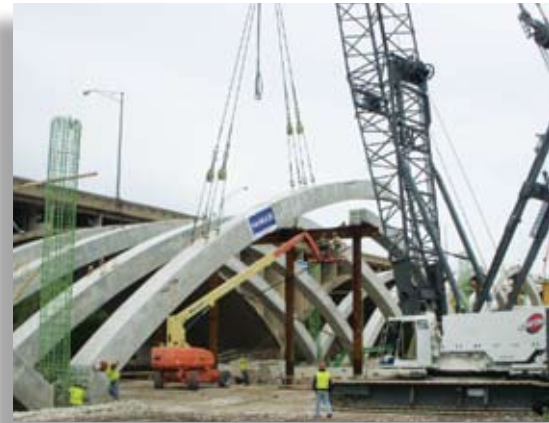
Precast concrete I-girders frame the approach spans and span between the spandrel bents. (top)
